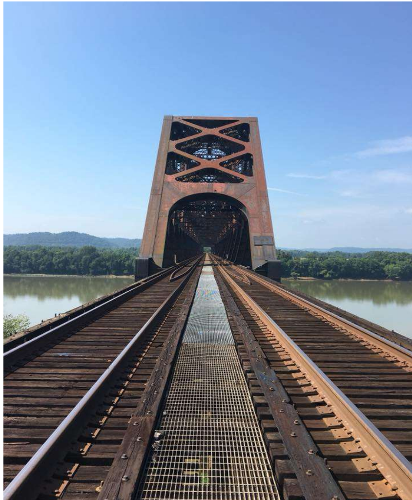
The Sciotoville Bridge. C&O's 1,550-foot span, 8.2 miles east of Portsmouth in Scioto County, carries the Russell Subdivision over the Ohio River. Completed in 1917, it is still the largest riveted through truss bridge in the U.S.
